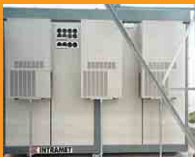
Free Cooling System
