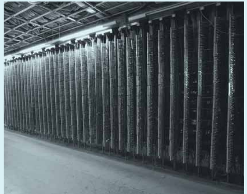
Digital Distributor (DDF – Digital Distribution Frame)
