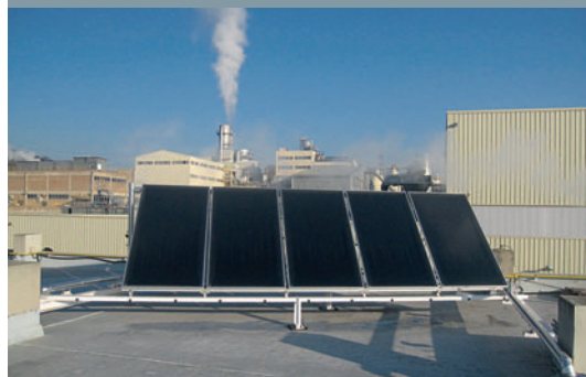
Pilot projects: In Spain, we have installed small-scale solar thermal systems at our sites in Seville and in Montornès (photo). These systems use the heat from solar radiation to provide hot water for the sites.
