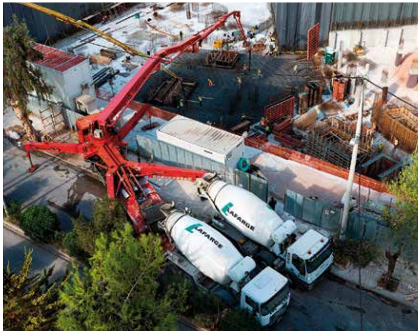
Concreting of Anangel Maritime Headquarters foundation in accordance to leed certification standards
