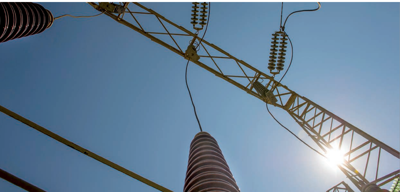
Energy supply, Catania, Italy
